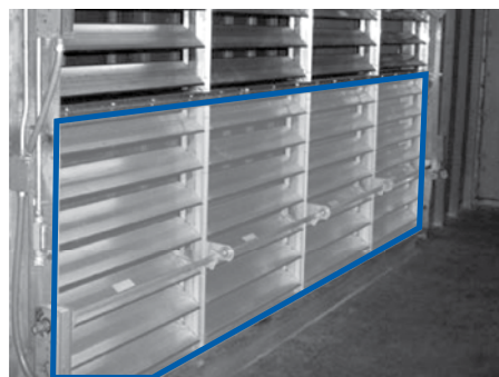
Return air dampers too big? Blanking them off may improve performance.
