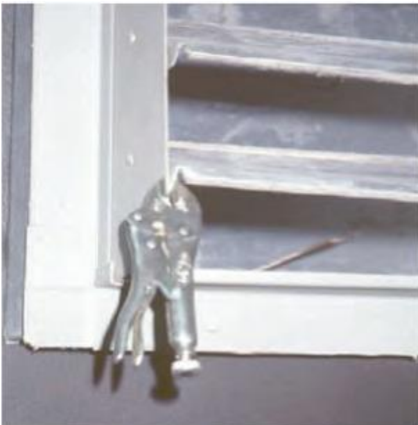
Figure 9.7.2. Damper quick fix – not recommended.
